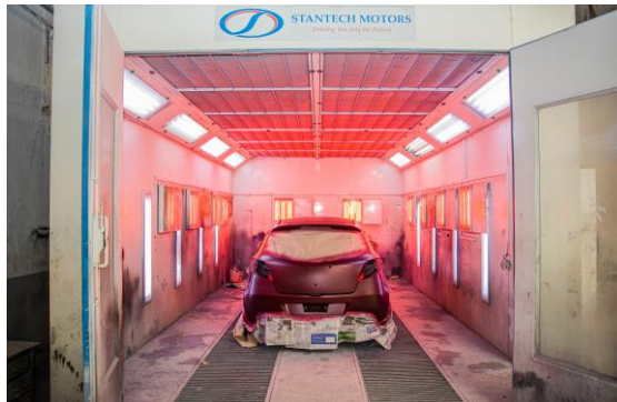
State of the Art Modern Spray Booth
