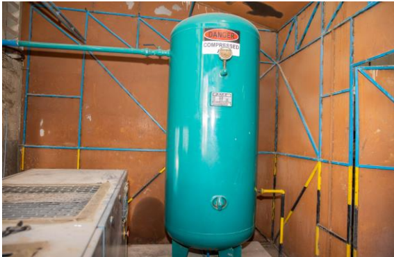
Compressor – Pressurized Air
